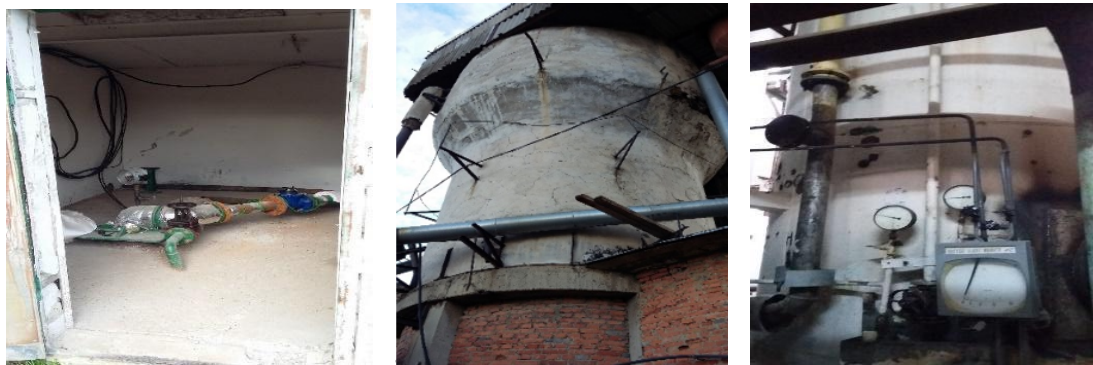
Figure 9: ground water intake and storage facilities
